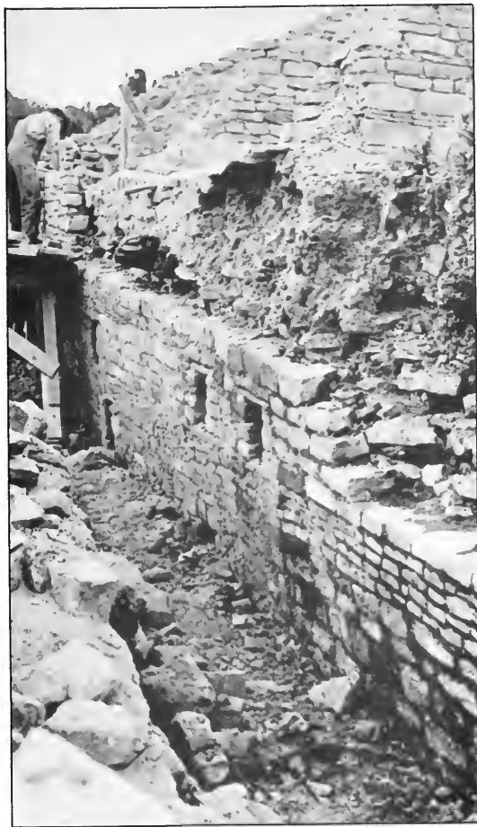
Figure 7.7. Resetting exterior wall of North Wing, 1934. Rubble core and shaped sandstone veneer evident.
